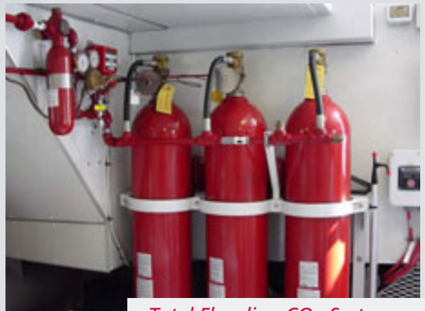
Total Flooding CO 2 System
